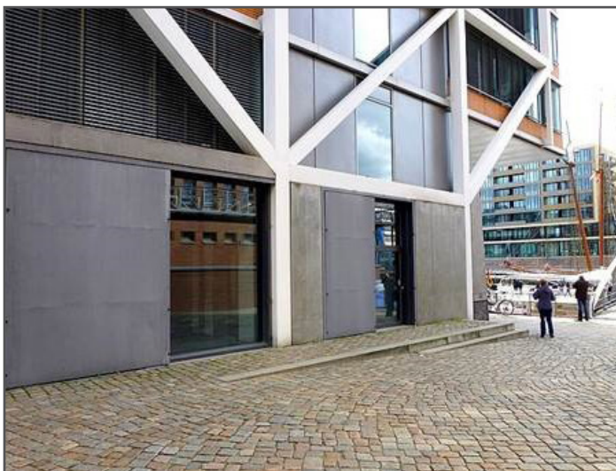
Ground floor windows designed to withstand high water pressures with steel bulkheads Source: Flooddefences.org. "Germany, Hamburg". Hafen City, Hamburg.
